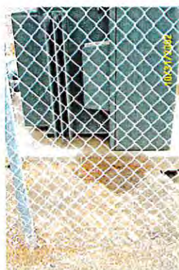
Stained Soil Underneath Pad-Mounted Transformer
