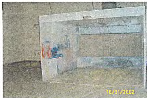
Water Wall Paint Spray Booth (Facing Northwest)
