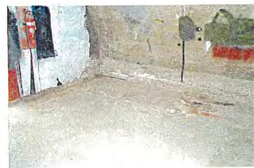
Interior View of Building 165 Showing Trench Drain and Paint Stain on Concrete Floor (Facing Northeast)
