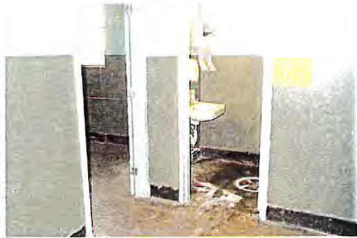
Restroom in Bldg. 46 and Location of Soil Sample Borehole HA5 and Drain Sample DS2 (Facing South)
