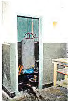
Utility Room with Service Sink and Location of Soil Sample Borehole HA2 and Drain Sample DS1 (Facing Northeast)
