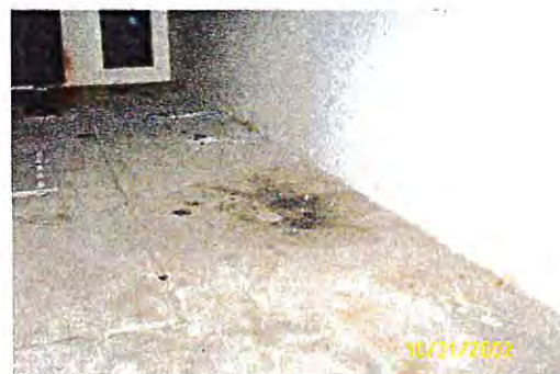
Interior of Test Cell Showing Plugged Floor Drain and Stained Concrete. Soil Sample Borehole HA2 was Drilled Next to Floor Drain (Facing Southeast)
