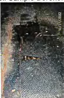
Staining around Trench in Service Bay Near Soil Sample Borehole HA1
