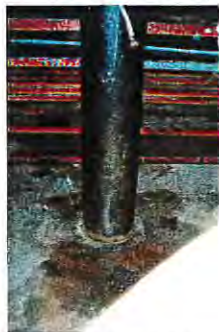
Staining around Hydraulic Hoist in Service Bay Near Soil Sample Borehole HA6
