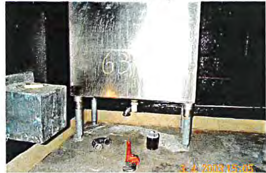
P-trap of Service Sink in X-ray Processing Room Where Drain Sample DS1 was Taken (Facing West)
