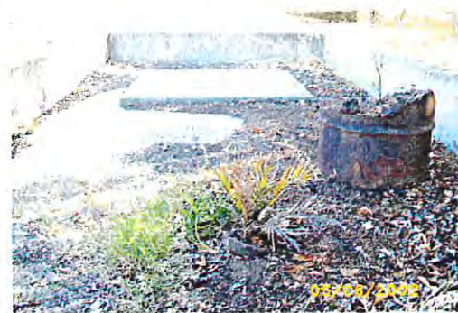
Foundation of Building 632 with Corroded Drum and Floor Drain in Foreground. Location of Soil Sample Borehole HA1 (Facing Southwest)
