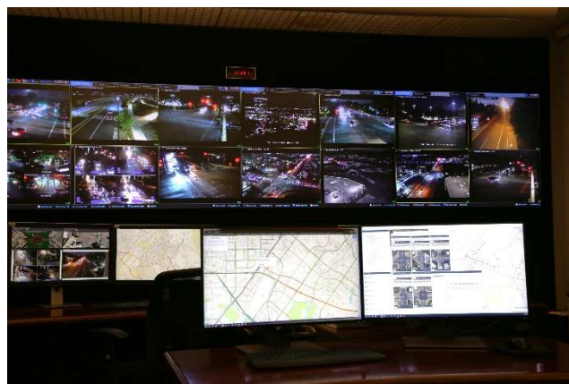
Traffic Management Center (TMC)
