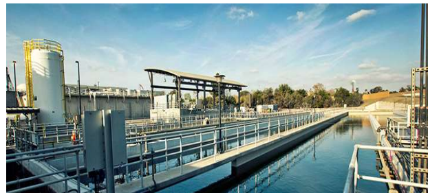
Michelson Water Reclamation Plant. Source: Irvine Ranch Water District
