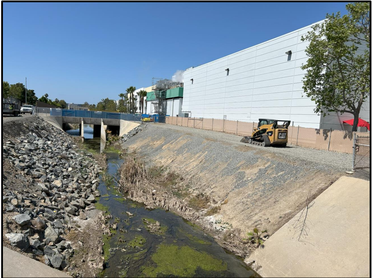
Figure 4.3-5 WEST BANK OF BARRANCA CHANNEL FROM SOUTH OF ALTON PARKWAK – TOWARD SMALL STREET CROSSING; VIEW TO THE SOUTHWEST
