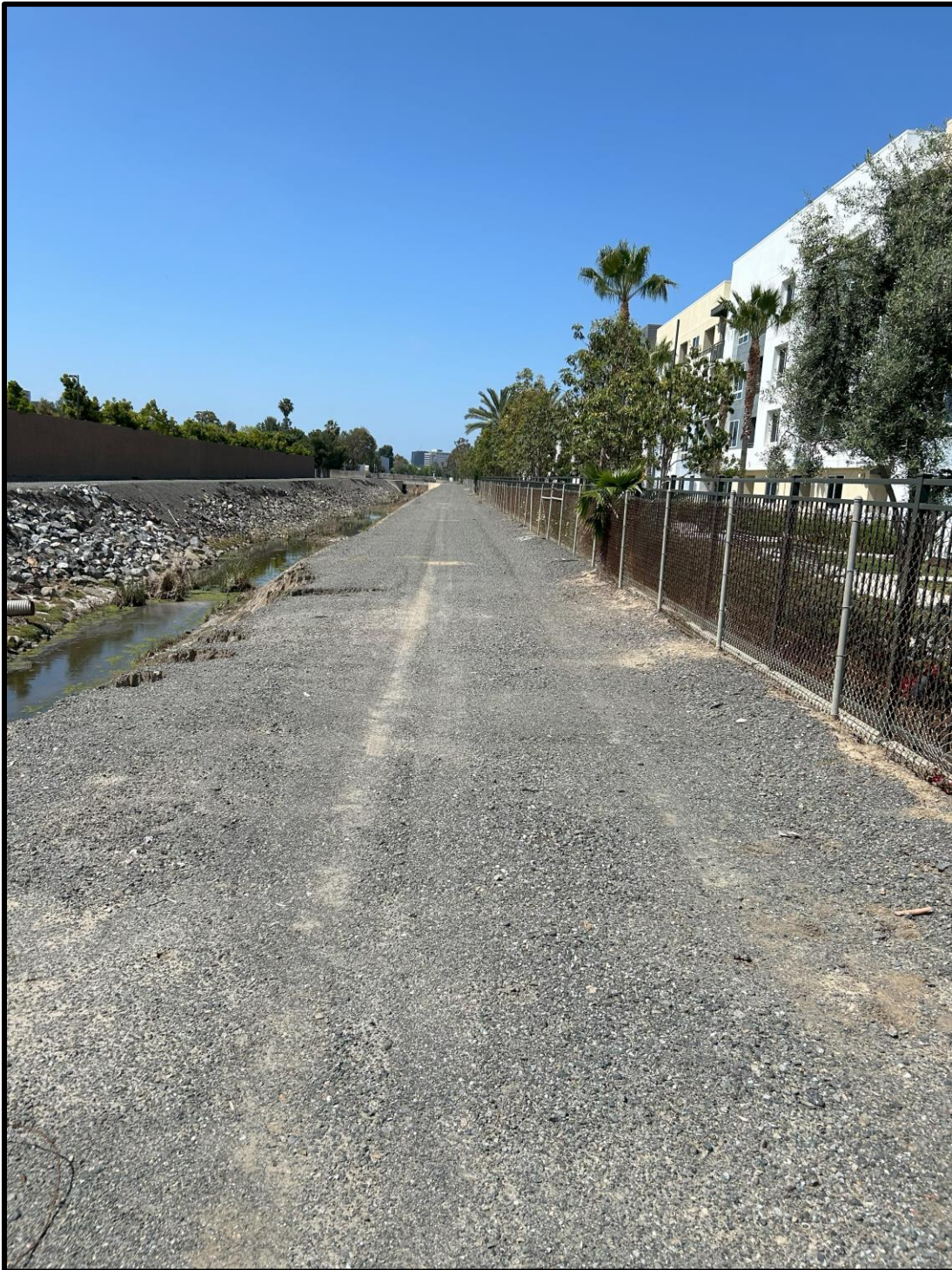
Figure 4.3-4 WEST BANK OF BARRANCA CHANNEL AND MAINTENANCE ROAD SOUTH OF MCGAW AVENUE; VIEW TO THE SOUTH
